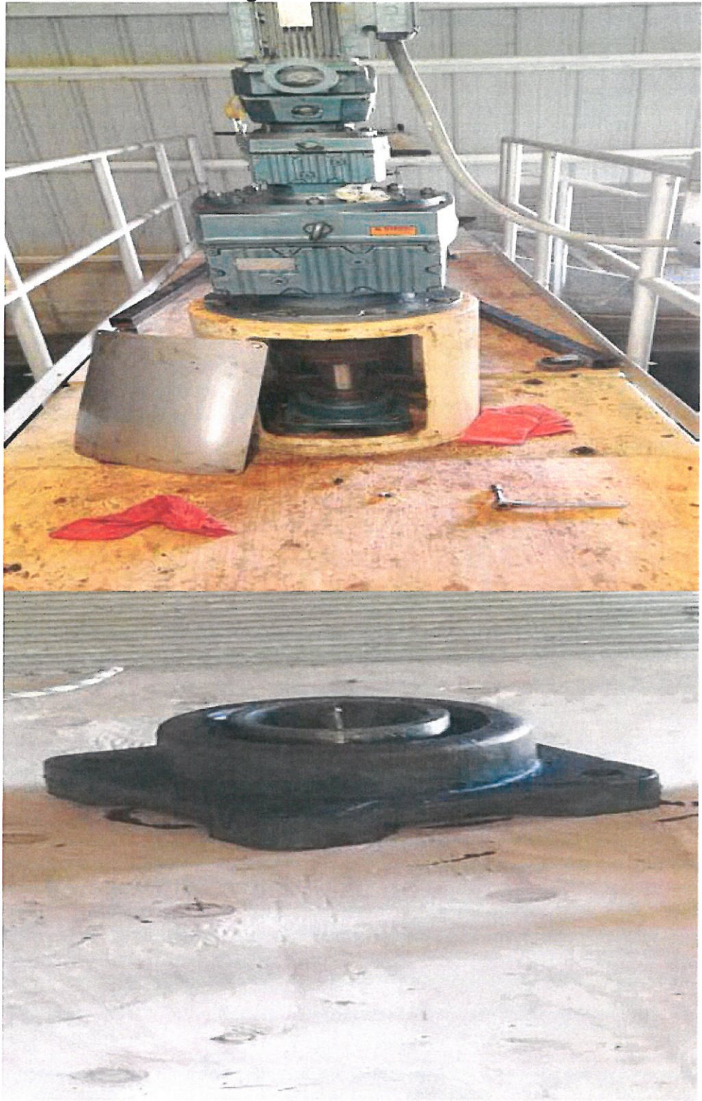
Flocculator and Bearing
