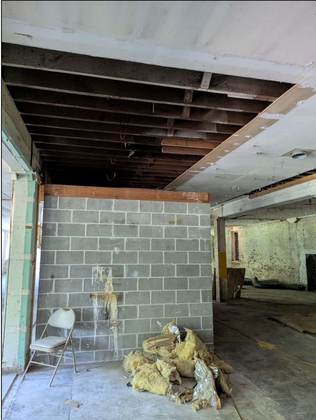
CEILING DAMAGE – DISREPAIR – MAIN FLOOR
