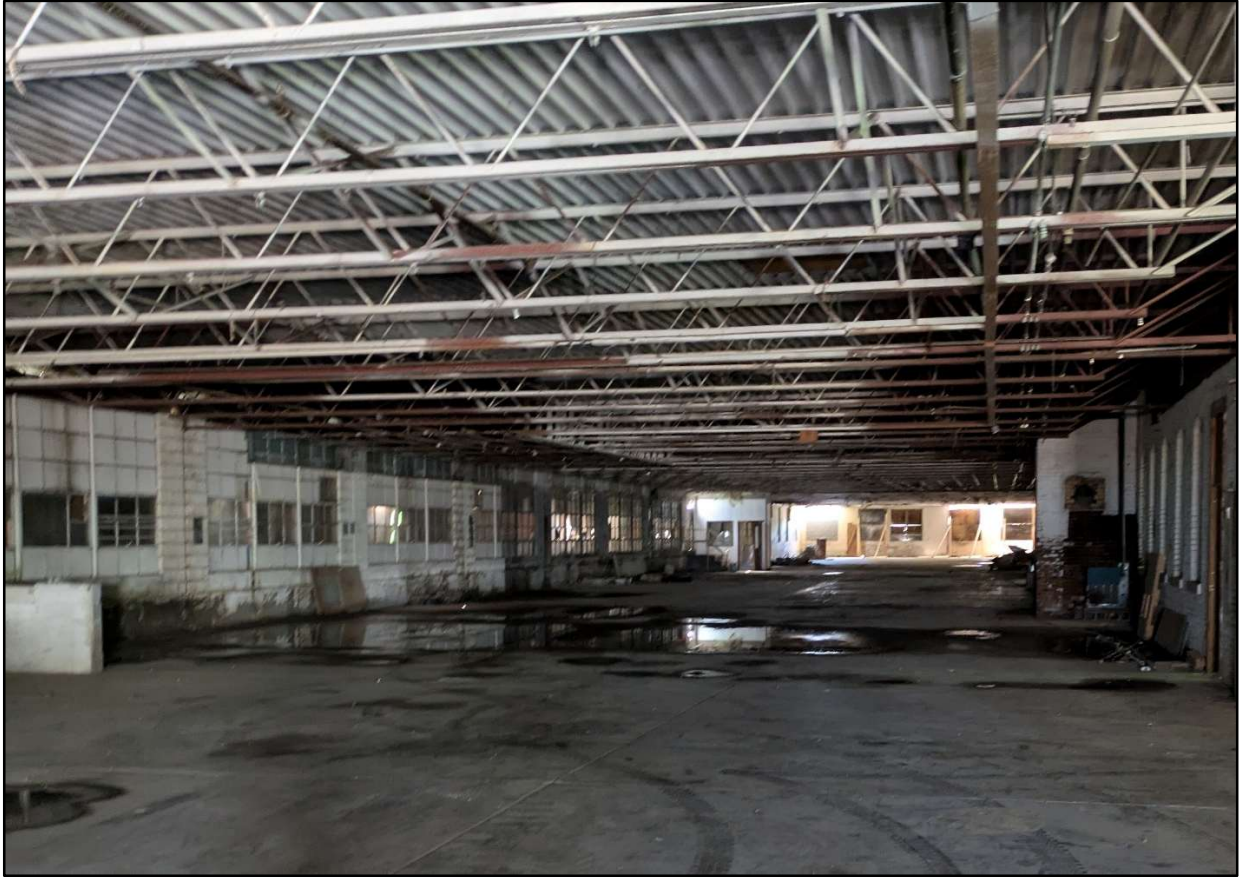
WATER INTRUSION – DISREPAIR – MAIN FLOOR
