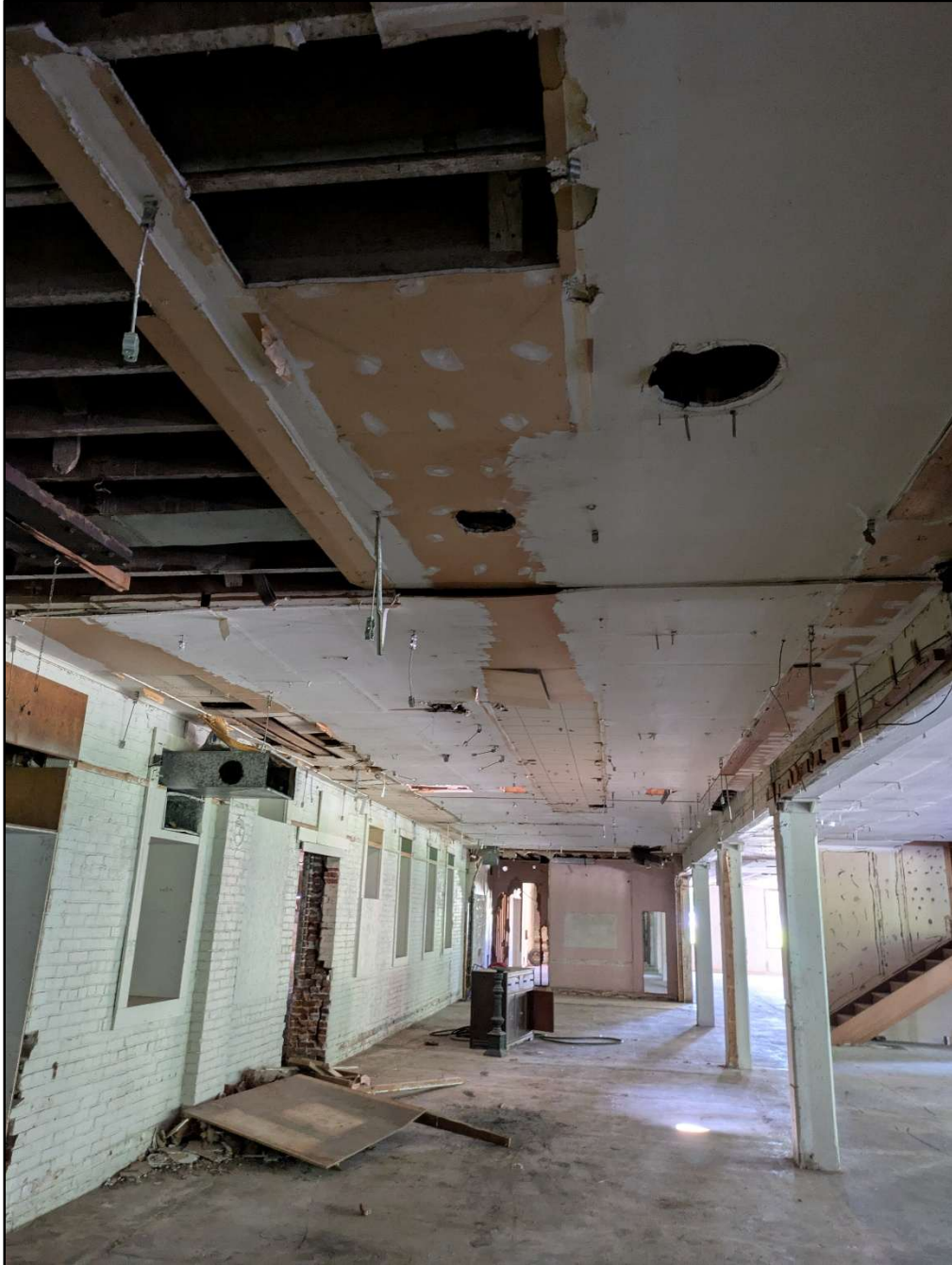
CEILING DAMAGE – DISREPAIR – MAIN FLOOR
