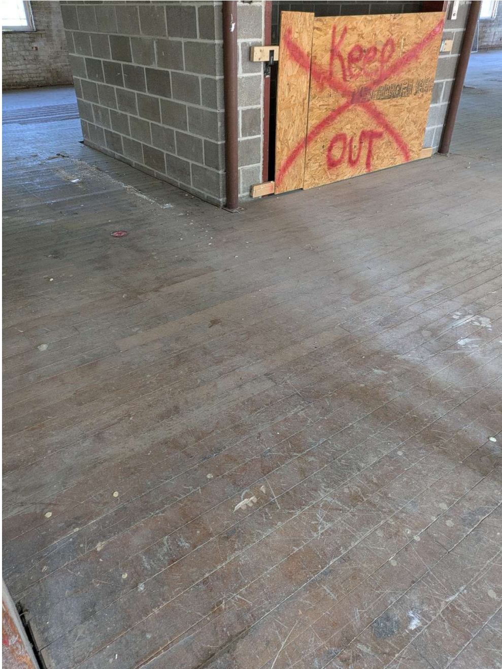
NON-FUNCTIONING FREIGHT ELEVATOR – DAMAGED FLOOR – SECOND FLOOR
