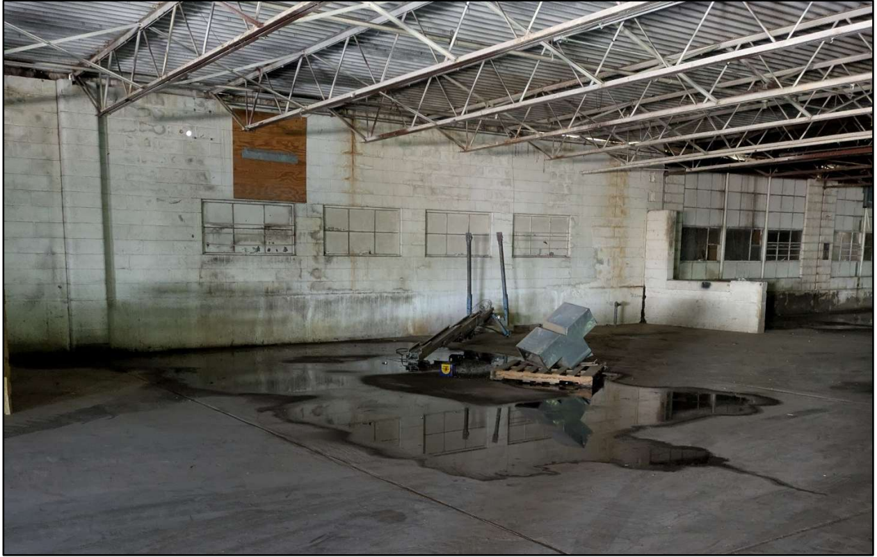
WATER INTRUSION – DISREPAIR – MAIN FLOOR
