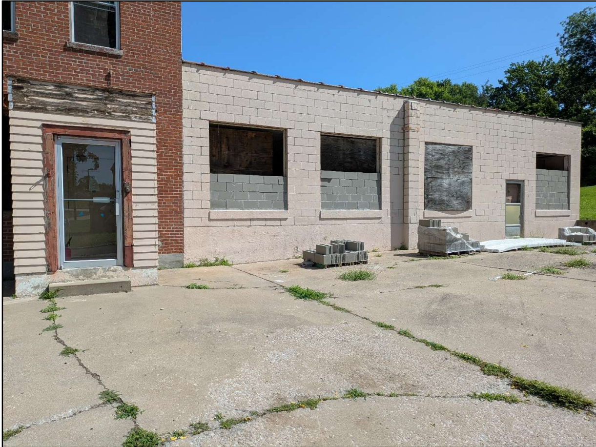
EXTERIOR DISREPAIR – SOUTH SIDE OF BUILDING – MAIN ENTRANCE
