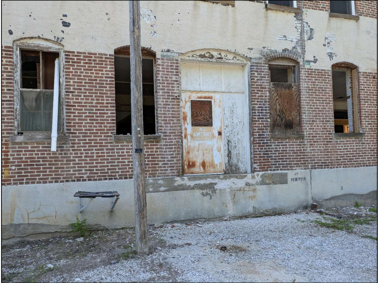
EXTERIOR DISREPAIR – WEST SIDE OF BUILDING
