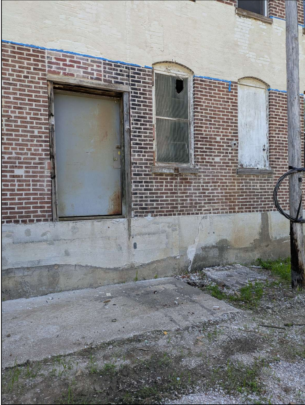
EXTERIOR DISREPAIR – WEST SIDE OF BUILDING
