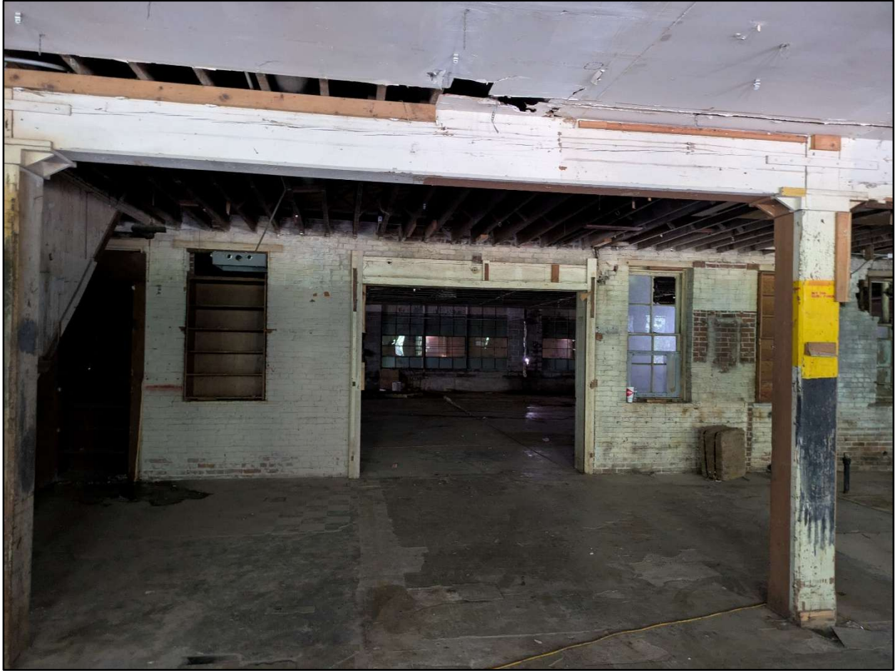
CEILING DAMAGE – DISREPAIR – MAIN FLOOR
